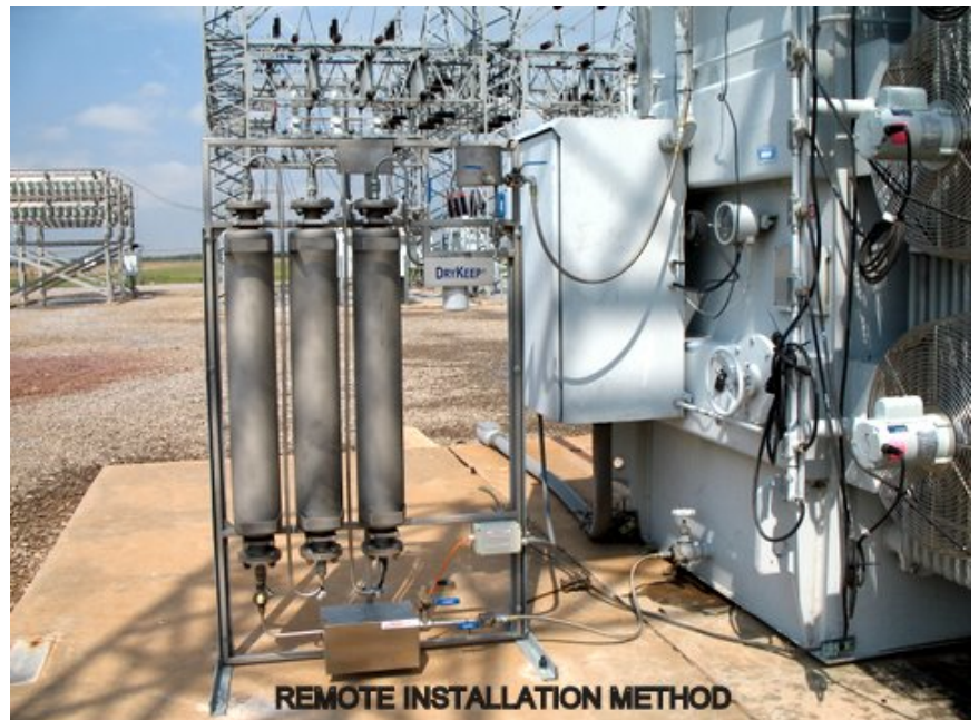
Figure 3: Installation adjacent to transformer on customer-fabricated free-standing frame
