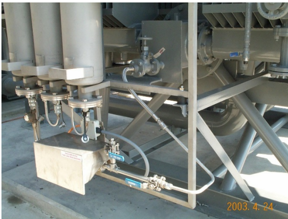
Figure 4: Connection from transformer to DryKeep® inlet valve.
