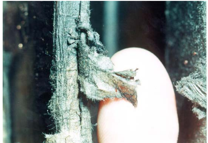
Decayed paper insulation
